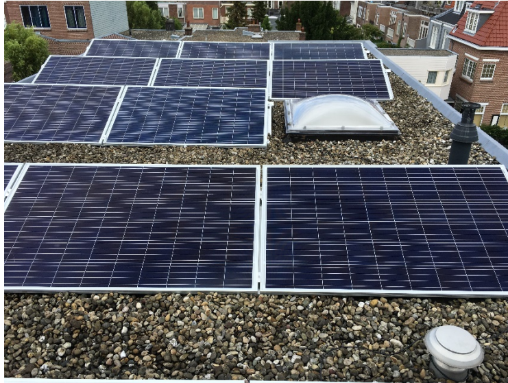
Figura 5.3 Paneles solares Haarlem Holanda (B. Oostenveld)
